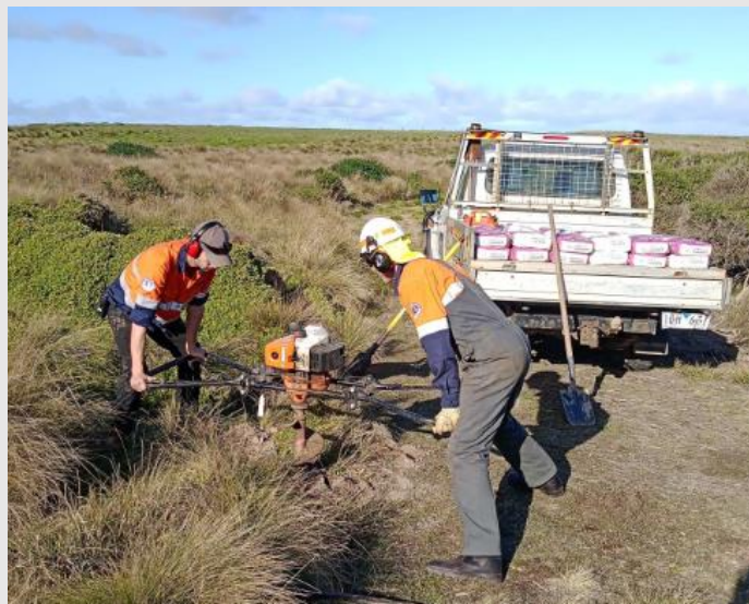
Management only signs bollards installed on the Fire break at Summerland Peninsula and managements track in the Five Ways reserve.
