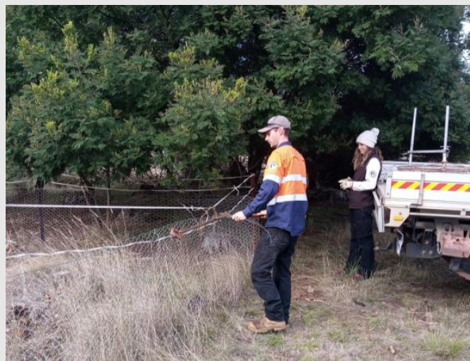
As part of the vegetation management program, Rangers Chris and Kat are seen working on fence maintenance at Five Ways Reserve.
